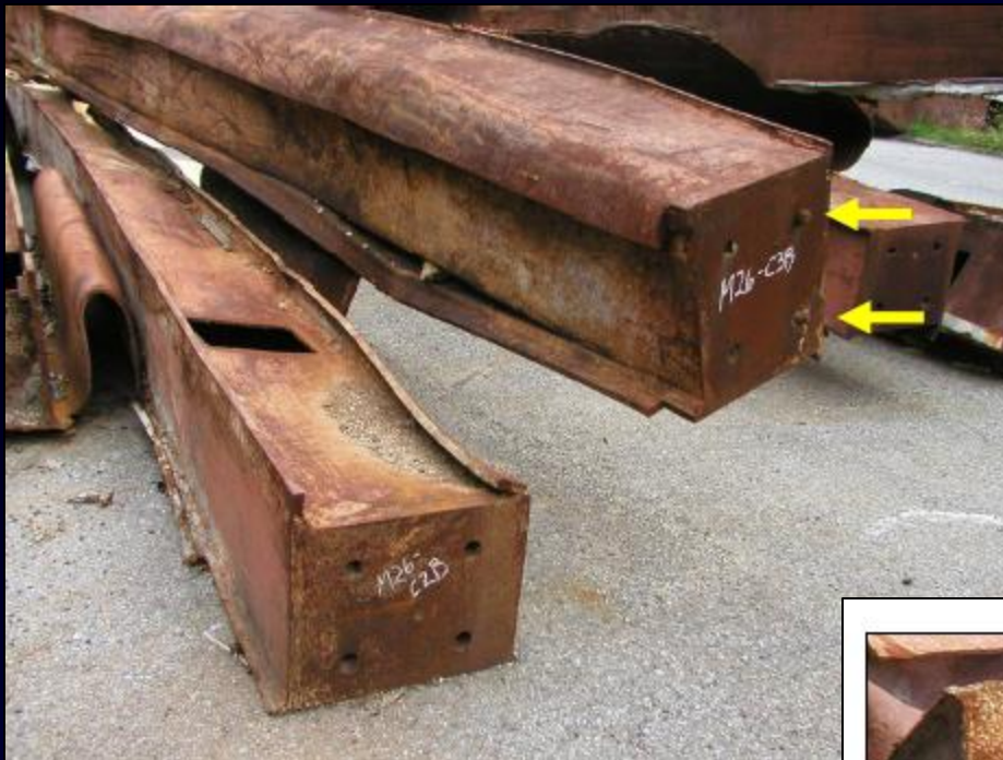
Figure 3-42, NCSTAR1-3C Perimeter columns from WTC 1 Floors 90-93
